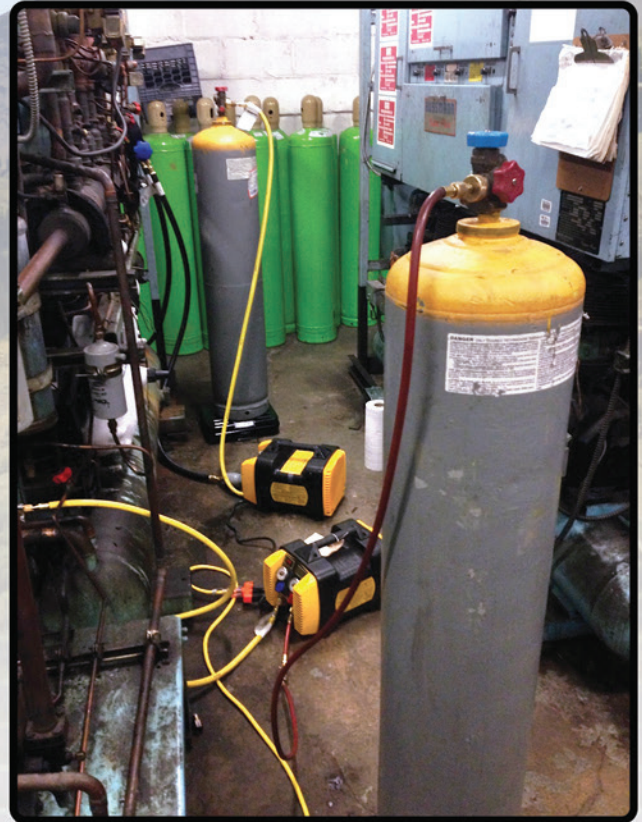
Above: On an R407A system retrofit of a low temperature ice cream case, the G5Twin recovered 600 pounds of R22 in record time, using the push-pull method.
