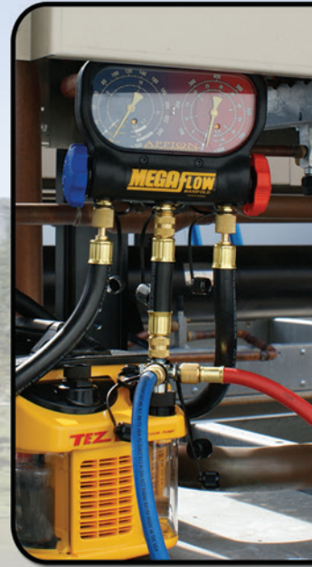
Above: At a large refrigeration job, a 30HP chiller went from atmospheric to 1,000 microns much faster than the previous method.
