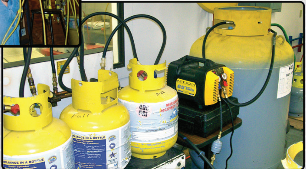
Above: G5Twin used daily in reclamation facility for tank transfer.
