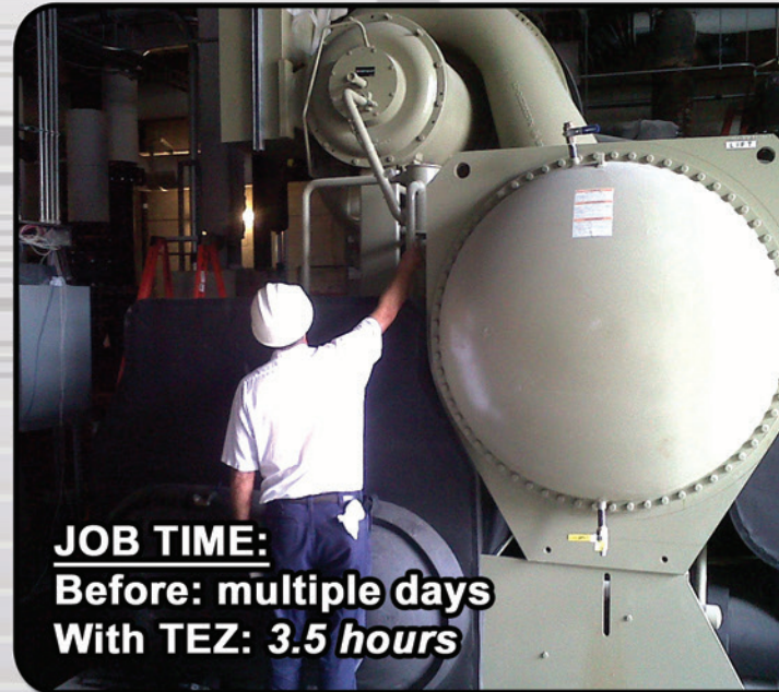
Above: This 2,000 ton chiller was pulled from atmospheric to 1,000 microns in only 3.5 hours, instead of days with a belt-driven pump.
