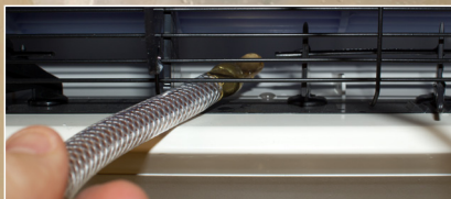
Clean inside the system
