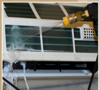
Clean coils from the front
